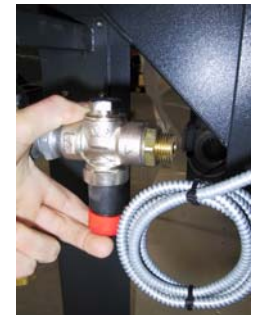
Sprinkler valve without hose
